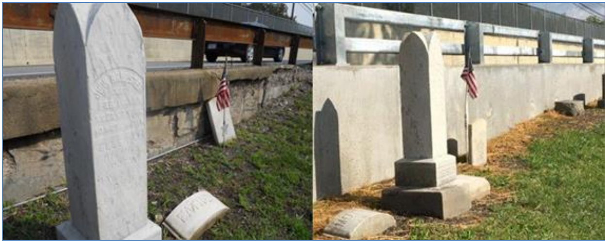
Frankstown Intersection project- A view of the same marker stones along the retaining wall before and after its replacement. Note that PennDOT right of way extends 6.5 feet beyond the face of the wall.
